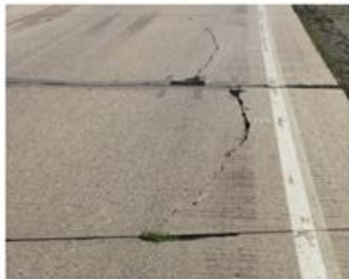
Figure 5 - Broken panels in Highway 60 East
