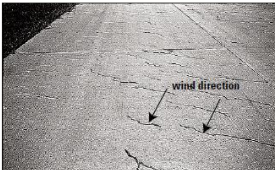
Figure 5-31. Deep plastic shrinkage cracks
